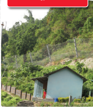
Rockfall Protection for Rangpo, India
