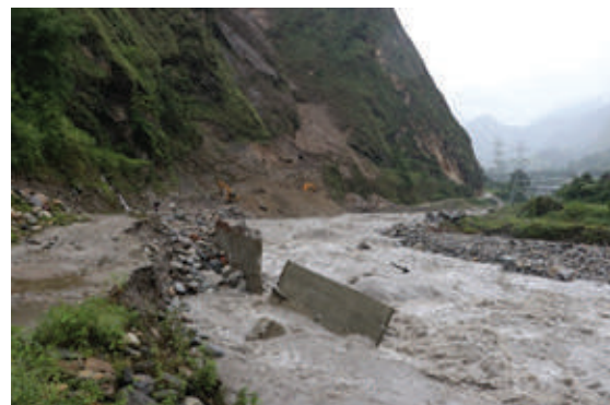
Figure 1: Consequence of the construction of road in the floodplain. An example from Kali Gandaki corridor road at Bhurung, Tatopani, Myagdi. The road was heavily damaged by the flash flood of July 20, 2020 with complete destruction to the R.C.C. shear wall.
