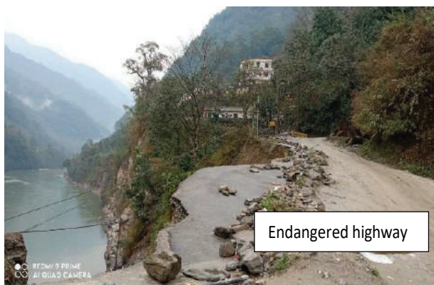
Fig. 1. Initial condition (a). at Site
