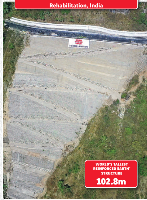
Tindharia Landslide Restoration and Rehabilitation, India
